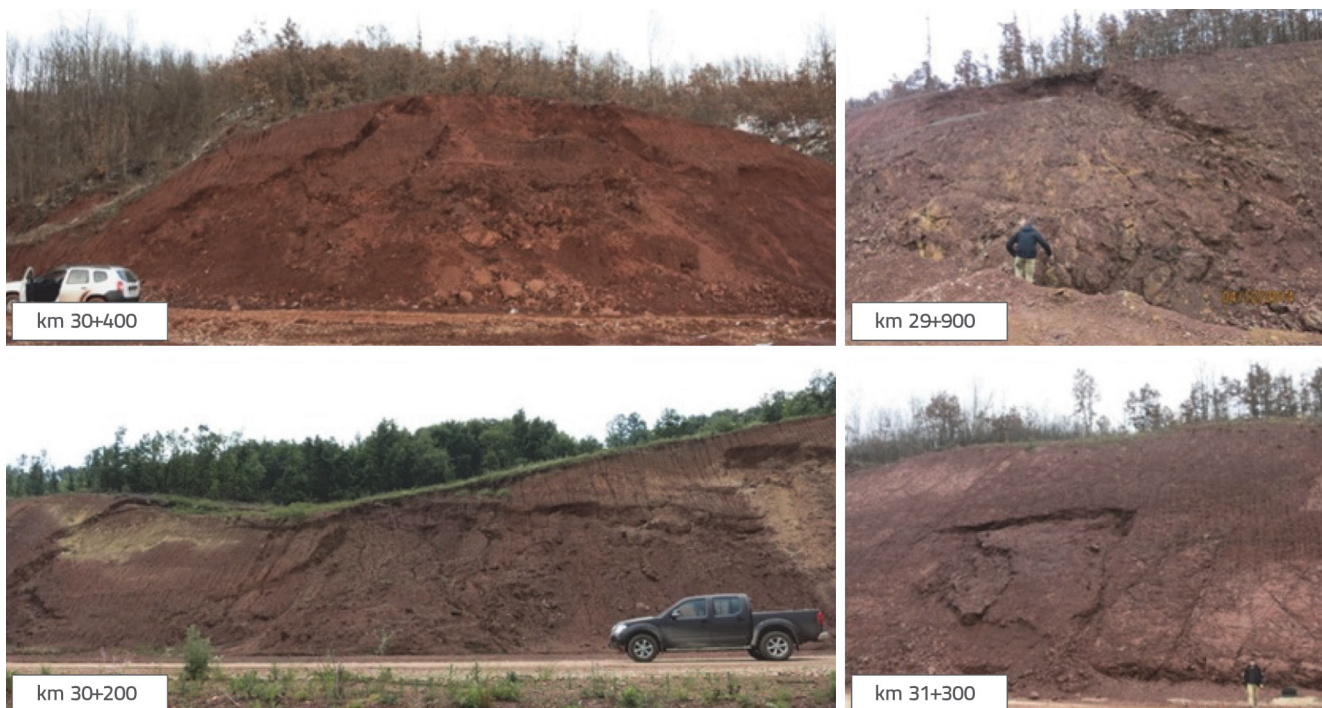
Figure 2. Typical failures in Permian shales and mudstones
